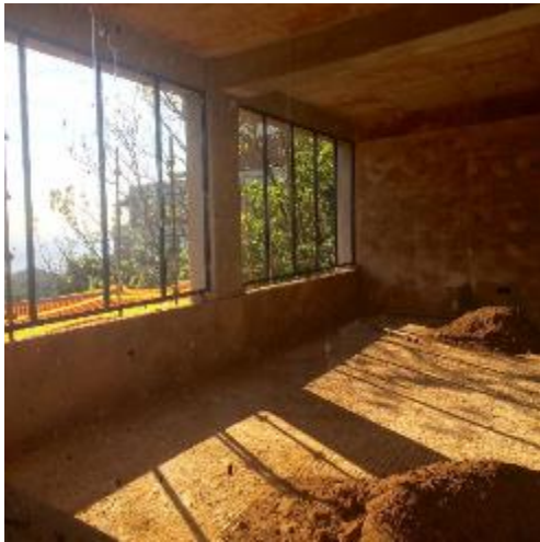
Figure 1: New office area with window frames installed, above gas cylinder storage area 1.
