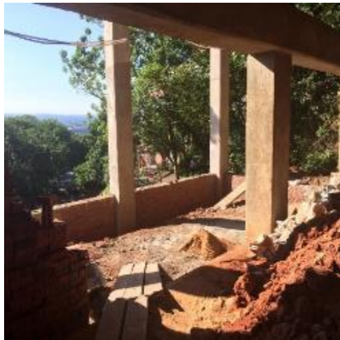
Figure 5: Gas cylinder storage area 1.
