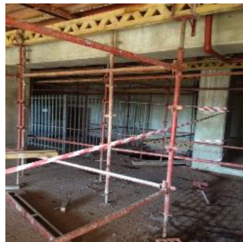
Figure 6: scaffolding spanning across the gas cylinder storage area 1 and area 2.
