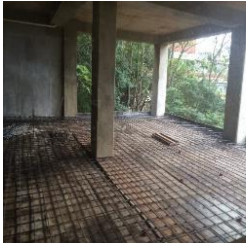
Figure 3: New slab foundation with grid layer (underpinning) View from the office window.
