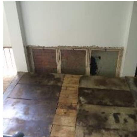
Figure 2: Windows behind the wall caused delays.
