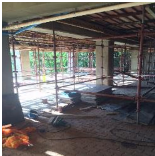
Figure 5: Gas cylinder storage area 1 with scaffolding. 20 May 2016
