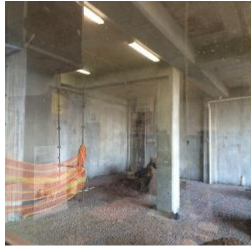
Figure 2: New office area closed up and plastered, above gas cylinder storage area 1.
