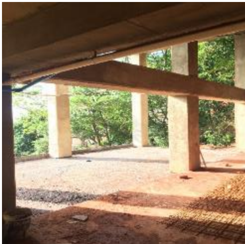
Figure 5: Gas cylinder storage area 1.
