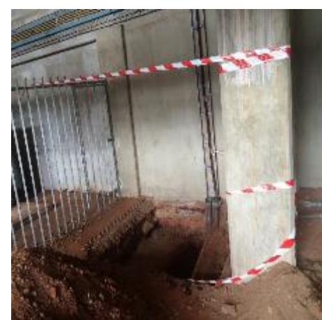
Figure 6: Gas cylinder storage area 2.
