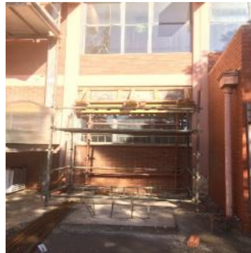
Figure 4: Wash station with hole and scaffolding staging.
