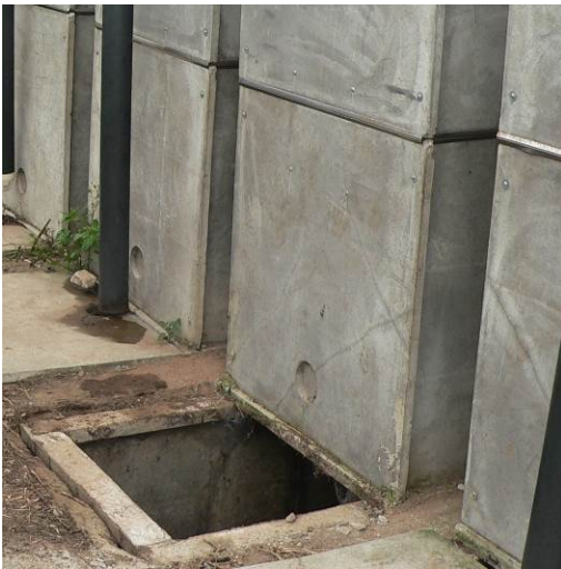
Ventilated Latrine School pits
