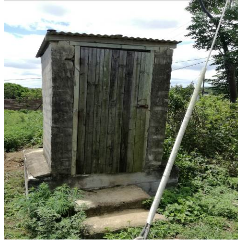
Urine Diversion toilets
