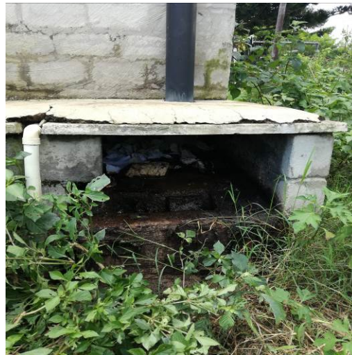
Urine Diversion toilets
