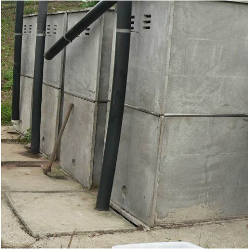
Ventilated Latrine School pits
