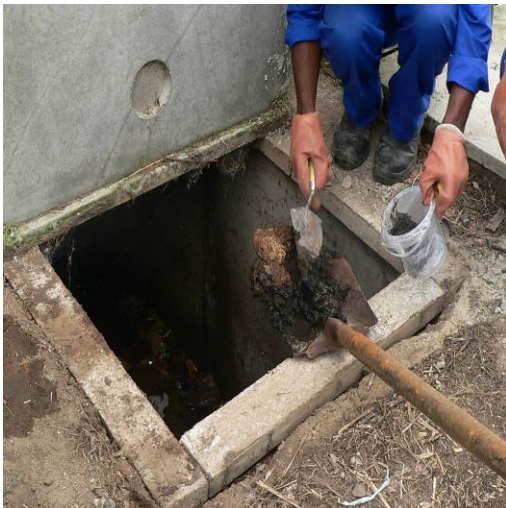
Ventilated Latrine School pits
