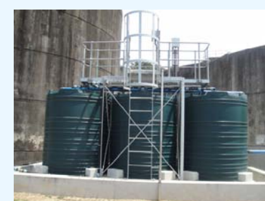
Effluent receiving and dosing
