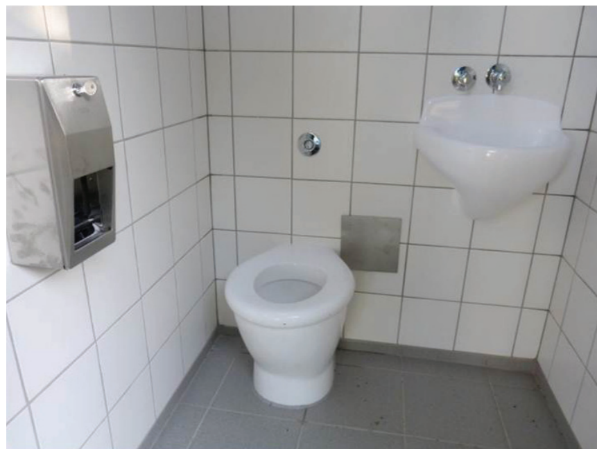
FIGURE 5 Inside a cubicle of an existing Hering toilet. Fixtures protrude through the back wall into the service corridor.
